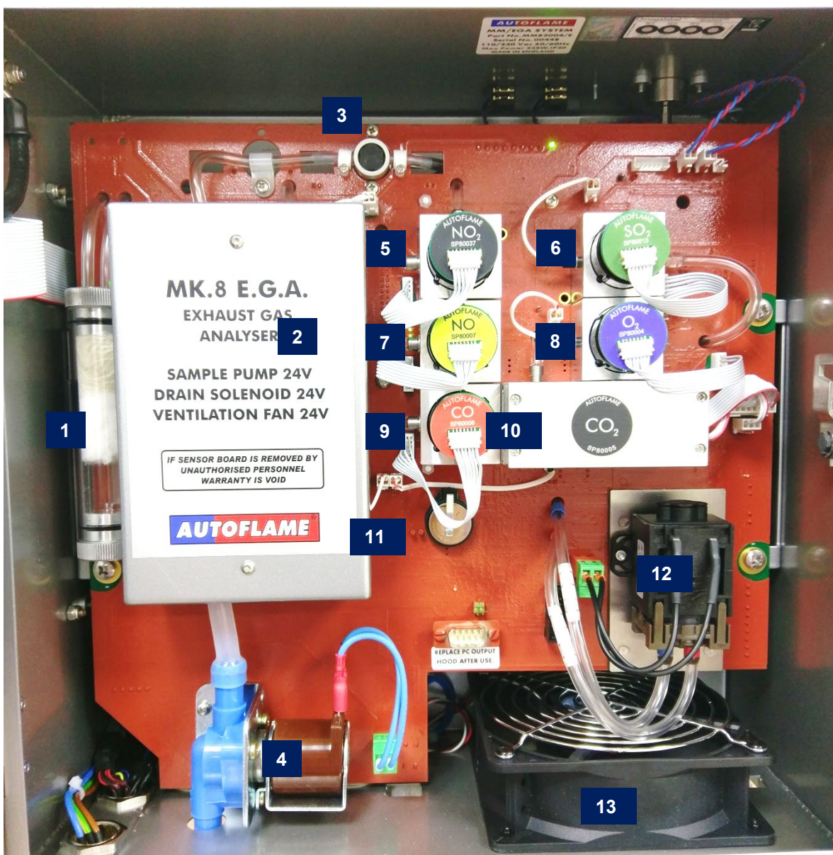
Figure 1.1.1.i Inside view of the EGA
